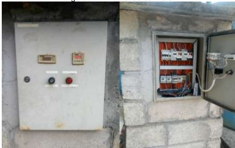
Figura 22 – Painel de controle
